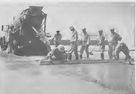
TO LEVEL the concrete, masons extend a board from one screed to another and move the concrete before them leveling and filling the area. PA NIVELA e concreto, muestanaran ta pone un pala pafo for di un lata pa otro y ta move e concreto cu e pala, asina nivelandu y yenand.
